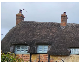
Figure 51: Thatch on a one-and-a-half storey building with a simple design and form.
