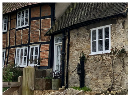
Figure 78: Metal rainwater goods.
