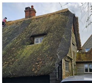
Figure 57: Thatch roof on the main house with clay tiled roof on the extension.
