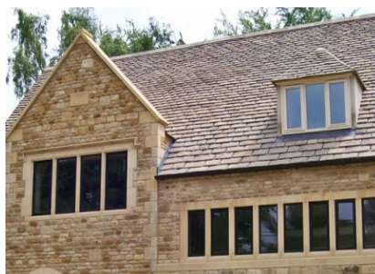
Figure 66: Stone walling and dressings with metal casement windows - modern version of Figure 65.
